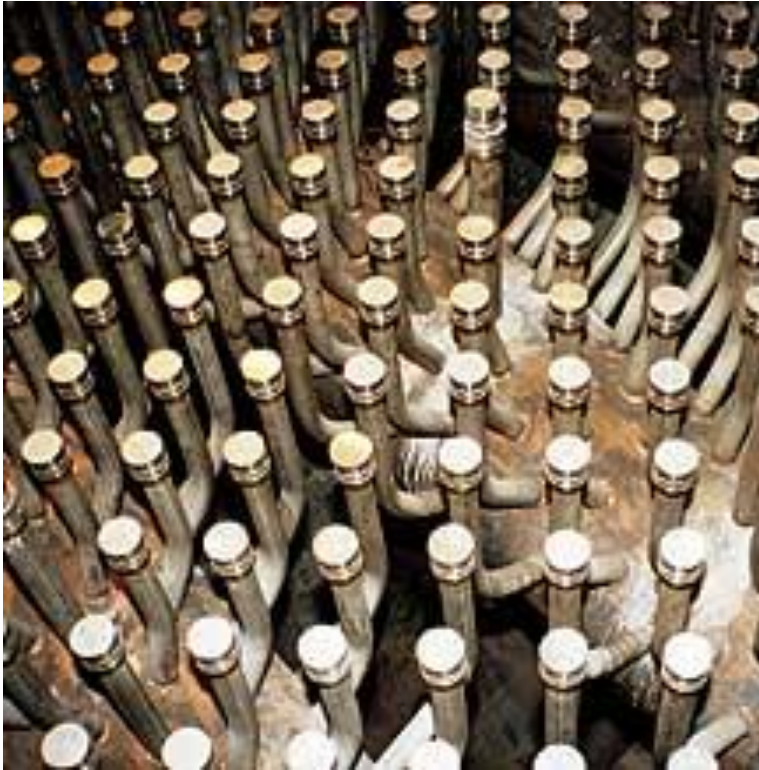
Grid of pipes
