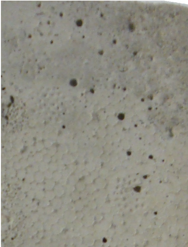
Figure 1: Air bubbles in the mortar surface
